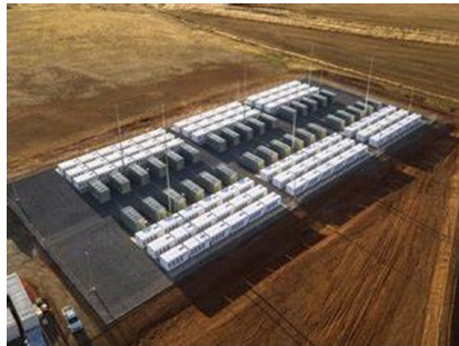
Hornsdale Energy Reserve Tesla 100 MW/129 MWh Jamestown - Austrália
