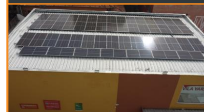
60. Vila Yara - 26,52 kWp
